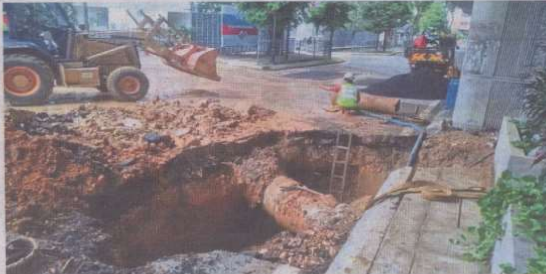
Work in progress: Syabas personnel repairing the burst underground pipe along Jalan Dewan Bahasa in Kuala Lumpur.
